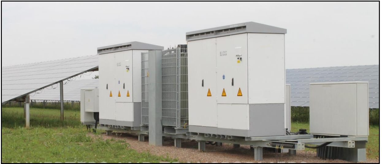
Figure 9d: Inverter and Sub-station Switchgear
