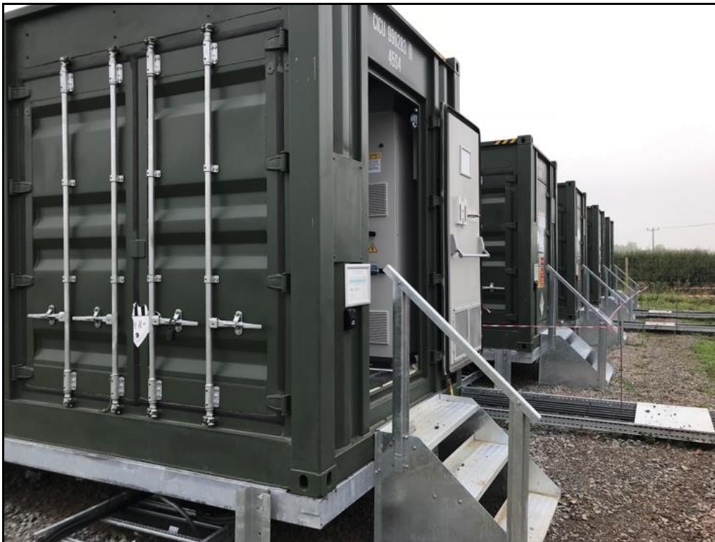
Figure 9e: Inverter, Battery and Sub-station Switchgear
