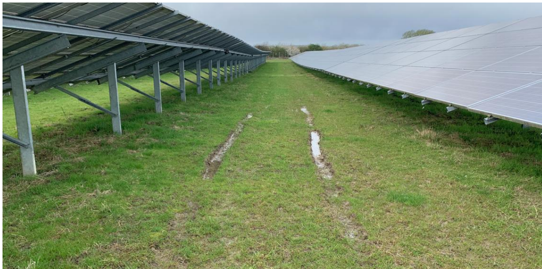
Photo 17: Example of minor ruts caused by vehicles
