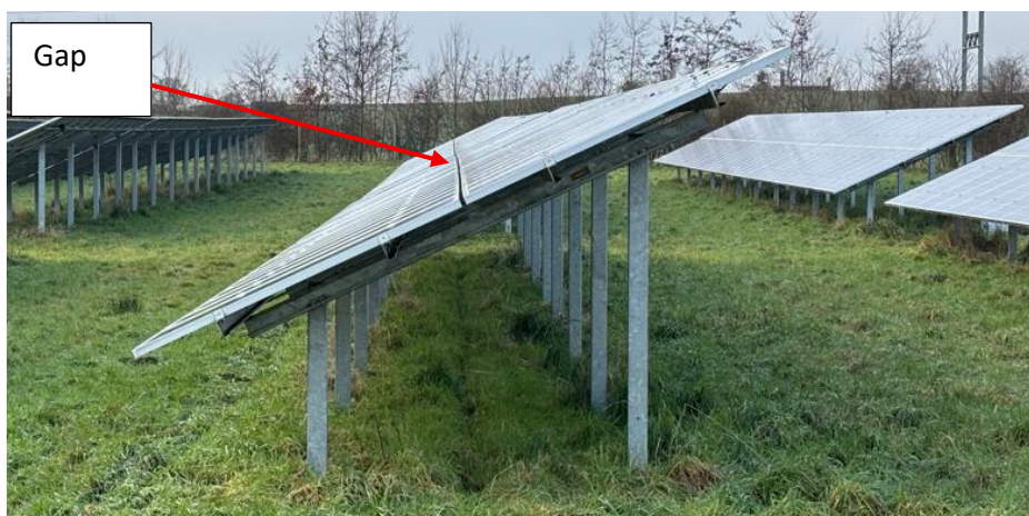
Photo 18: Panels array showing gaps between panels and between rows of panels
