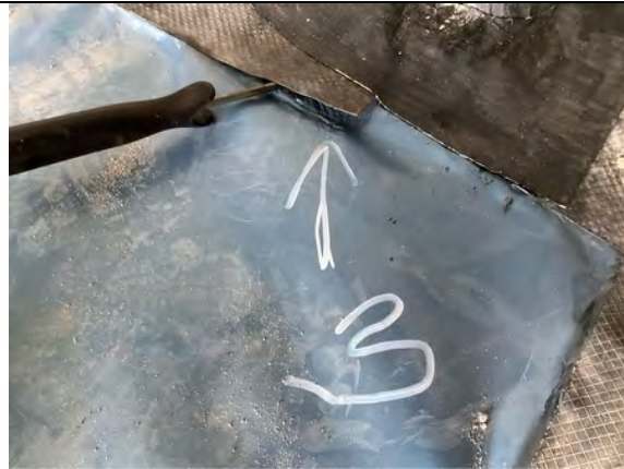
Plot 4. Recorded Defect.
