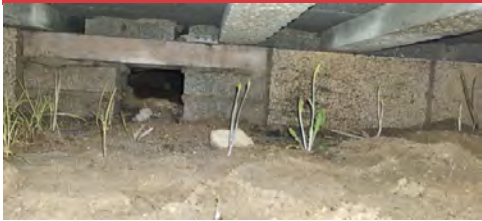
PLOT 1 - MISSED BLOCKWORK TO SLEEPER WALLS
