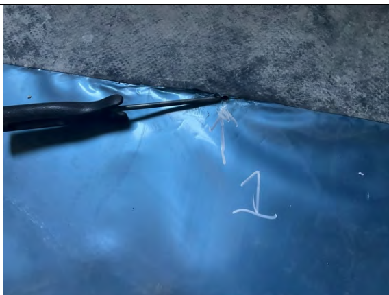
Plot 1. Recorded defect.
