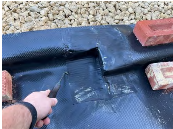
Plot 5 Garage. Probe testing to door threshold detailing.
