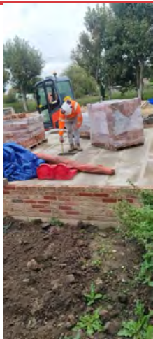
PLOT 5 GARAGE - CONFIRMATION OF VOID DEPTH
