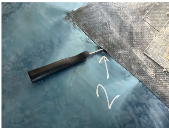
Plot 1. Recorded defect.
