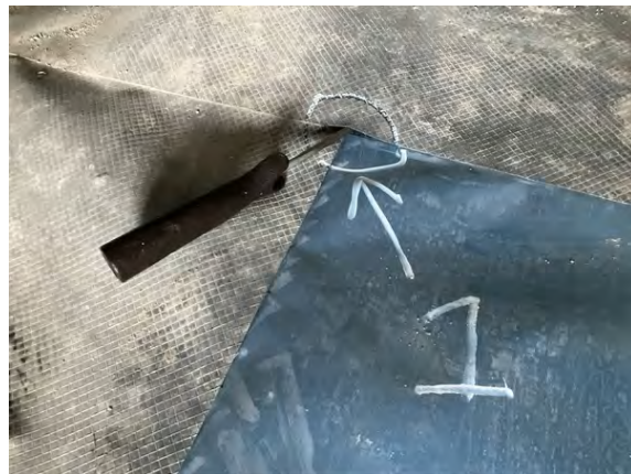
Plot 4. Recorded Defect.
