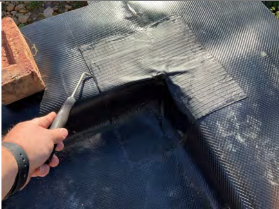
Plot 1. Probe testing to corner detailing.
