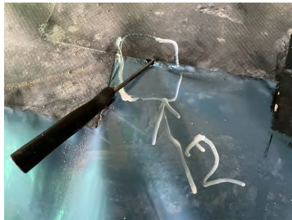
Plot 4. Recorded Defect.
