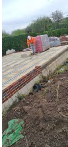
PLOT 3 GARAGE - CONFIRMATION OF VOID DEPTH
