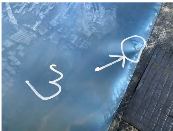
Plot 1. Recorded defect.
