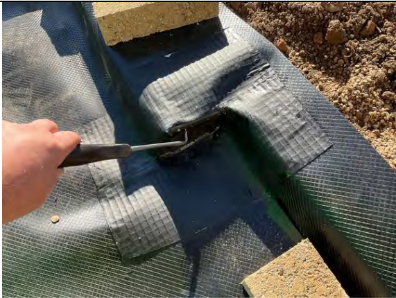
Plot 1 Garage. Probe testing to door threshold detailing.
