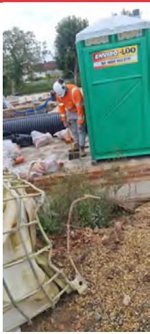
PLOT 1 GARAGE - CONFIRMATION OF VOID DEPTH
