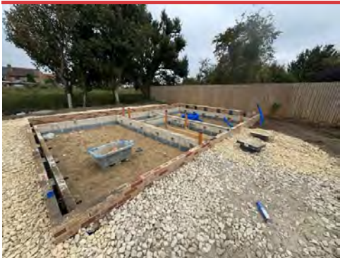
PLOT 5 - VOID DEPTH ~500MM, MISSED BLOCKWORK TO SLEEPER WALLS
