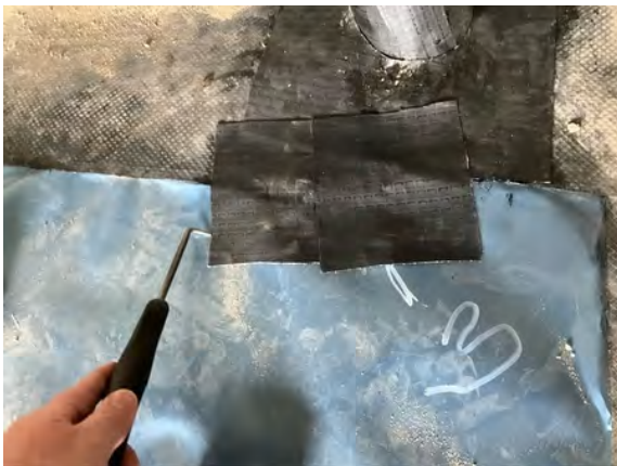
Plot 4. Defect was patched repaired using Juta GP1 SAM and then probe tested.
