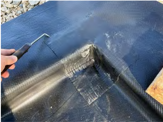
Plot 5. Probe testing to corner detailing.
