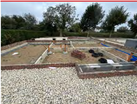
PLOT 3 - VOID DEPTH ~500MM, MISSED BLOCKWORK TO SLEEPER WALLS
