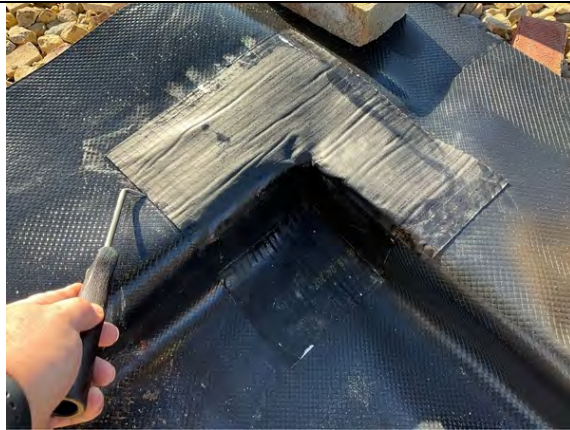
Plot 3. Probe testing to corner detailing.
