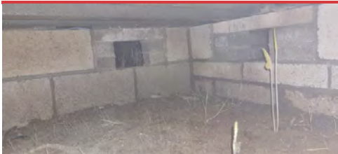
PLOT 4 - MISSED BLOCKWORK TO SLEEPER WALLS
