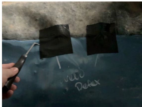
Weld defects patch repaired by MEC using Juta GP1 SAM, heat and pressure applied – probe tested.
