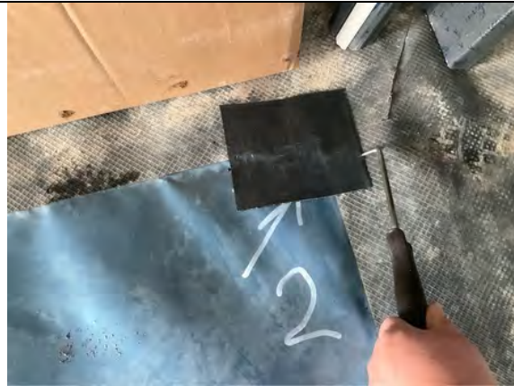
Plot 5. Defect was patched repaired using Juta GP1 SAM and then probe tested.
