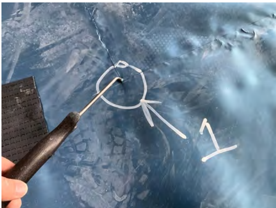
Plot 5. Recorded Defect.
