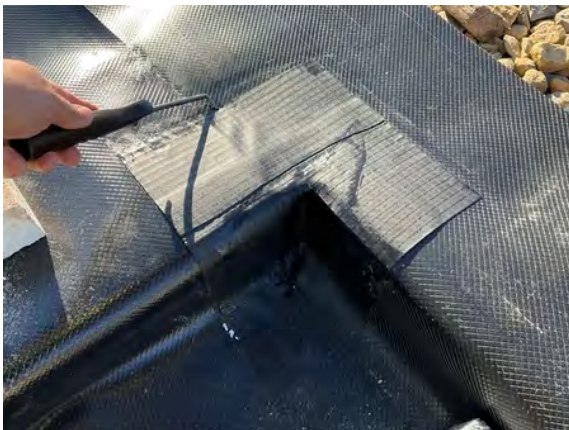
Plot 4. Probe testing to corner detailing.
