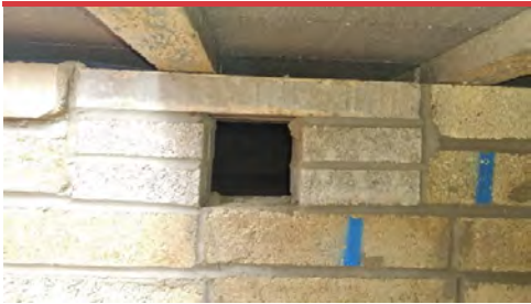
PLOT 2 - MISSED BLOCKWORK TO SLEEPER WALLS
