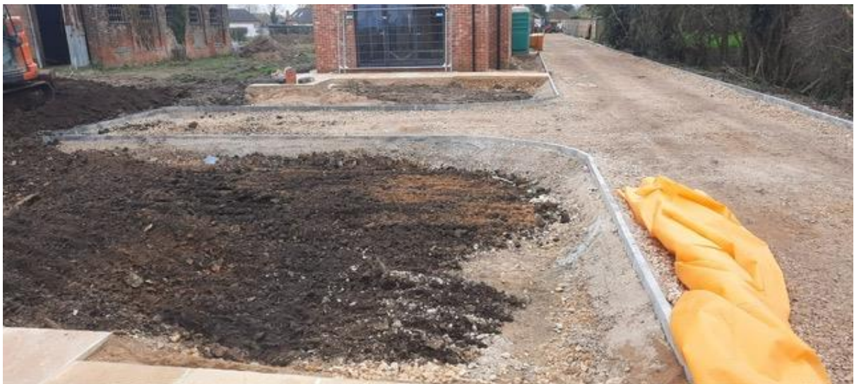
Plot 4 Installation Photographs
