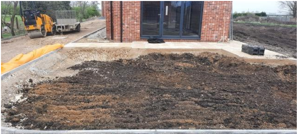
Plot 3 Installation Photographs
