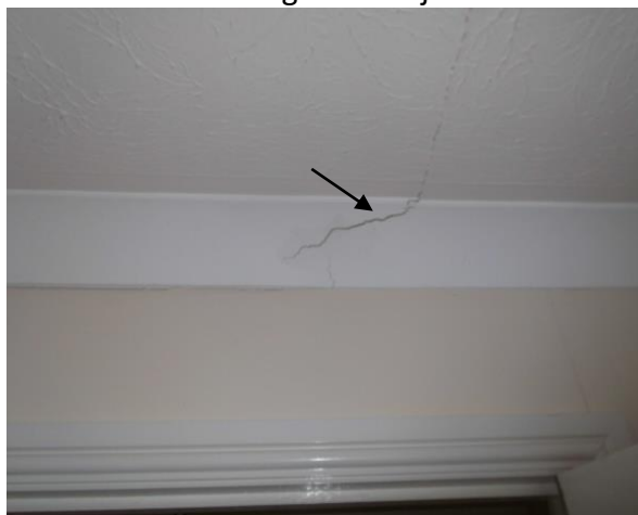
Cracking above rear left hand bedroom door way onto landing
