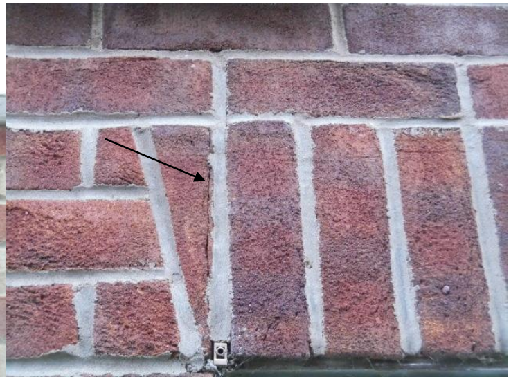
Minor cracking above left hand lounge/diner window
