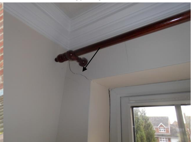
Cracking to front right bedroom window
