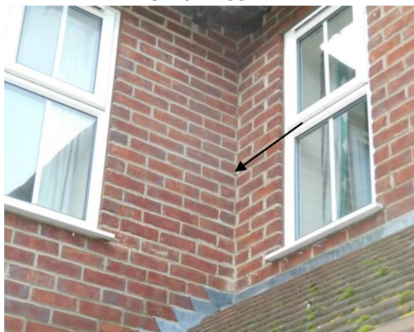
Minor cracking at front junction
