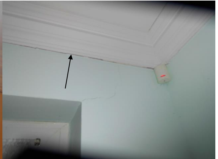
Cracking above front door to hallway
