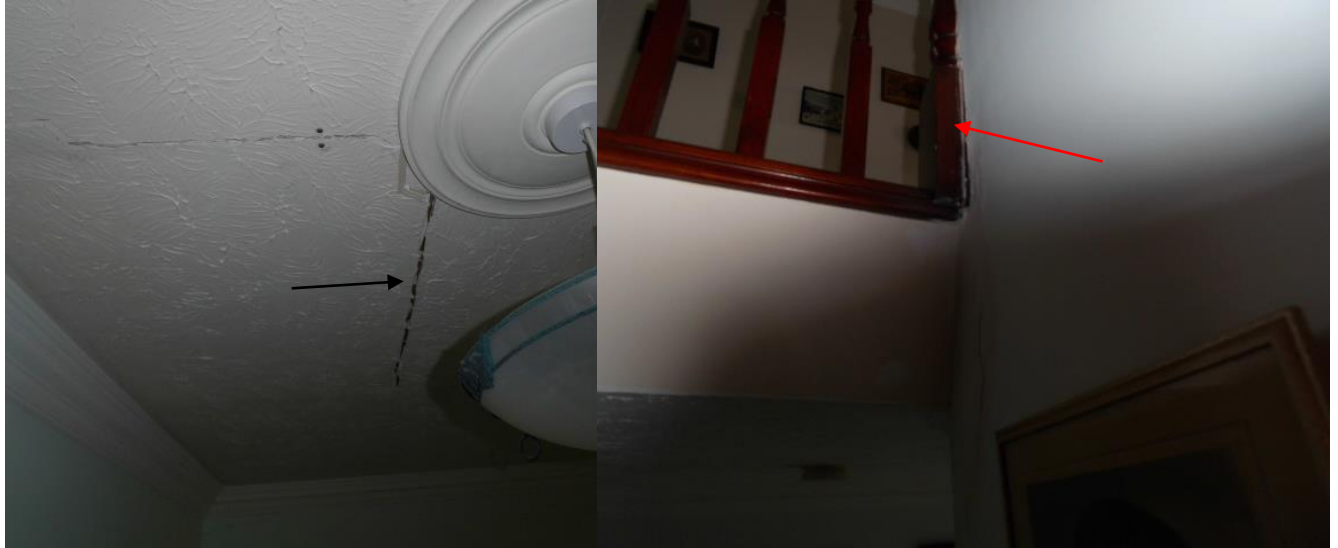
Landing – cracking to ceiling
