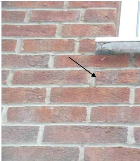
Minor cracking below left hand ensuite window
