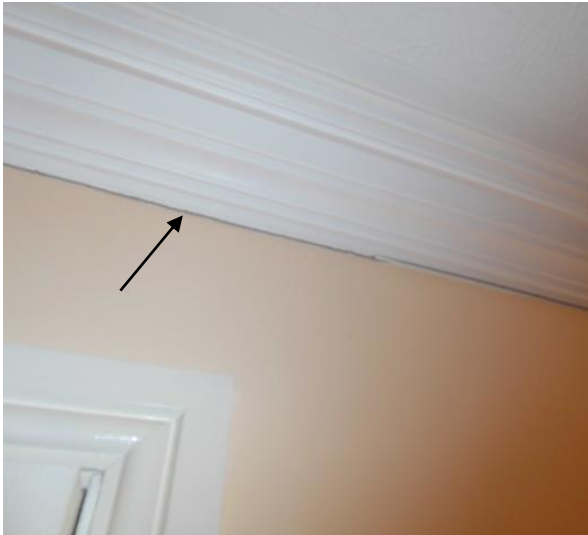
Cracking between wall and coving to lounge/diner
