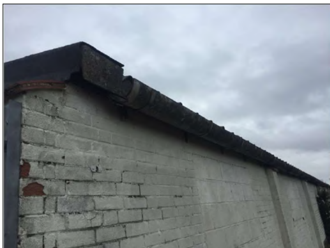
G – View of possible asbestos containing guttering.
