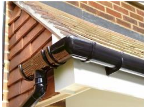
Black & Zinc Rainwater Pipes
