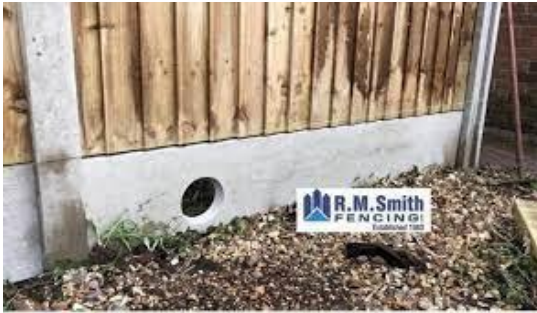
Holes within concrete gravel-board
