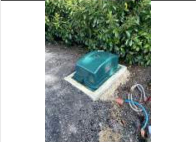
09: Package Treatment Plant (PTP) installed and located within the northeast of the Site
