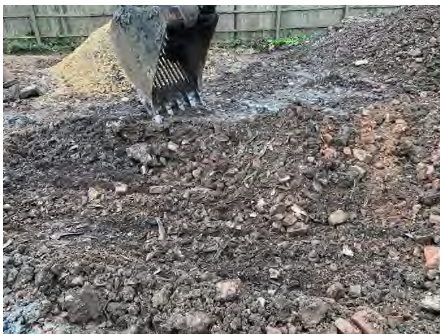
Plate 41: Asbestos cement tile fragments encountered in upper 0.5m of Hotspot B (BH206) remedial excavation
