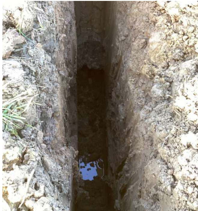
Photo 3: TP02A, showing water ingress.
