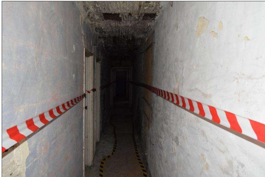
Plate 29 (shot 243): View down the corridor on second floor, showing area of removed plaster on the ceiling. Looking west
