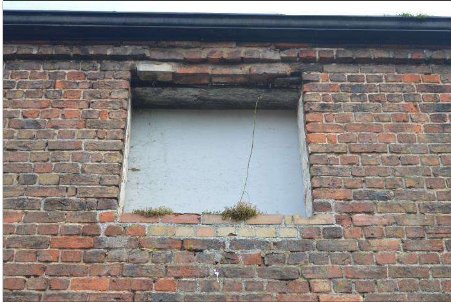
Plate 54 (shot 49): Representative view of boarded pitching hole on first floor. Looking east-southeast
