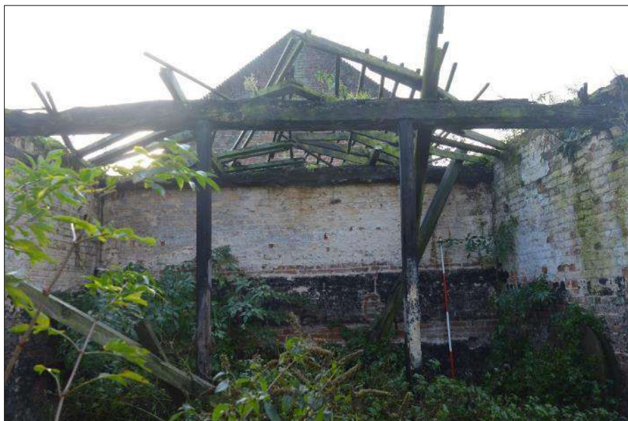
Plate 61 (shot 38): General view of C0.1 showing collapsed rafters. Looking south-southwest, 2m scale
