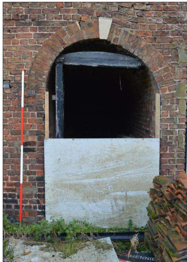
Plate 57 (shot 56): Slumping archway. Looking east-southeast, 2m scale
