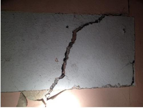
Structure 1- crack in wall on first floor
