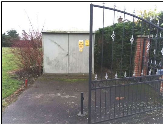
Sub station in northwestern corner of larger southern site.
