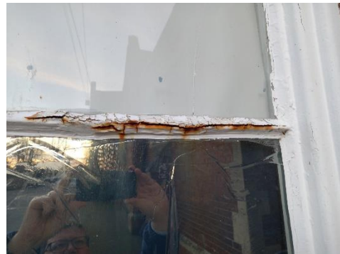
Figure: 8 Location: Original Building Defect: Life expired and dilapidated timber windows
