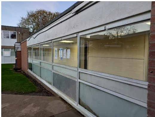
Figure: 9 Location: English Block Defect: Aged and life expired steel windows
