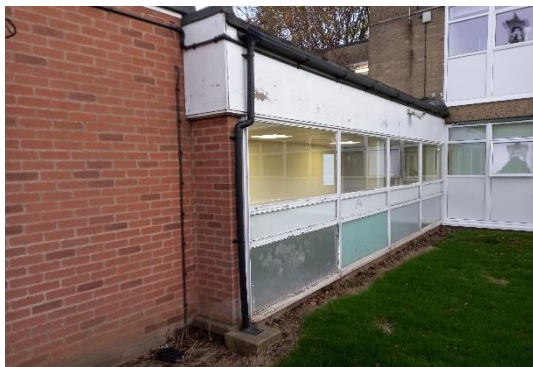
Figure: 11 Location: English Block Defect: Aged and life expired steel windows
