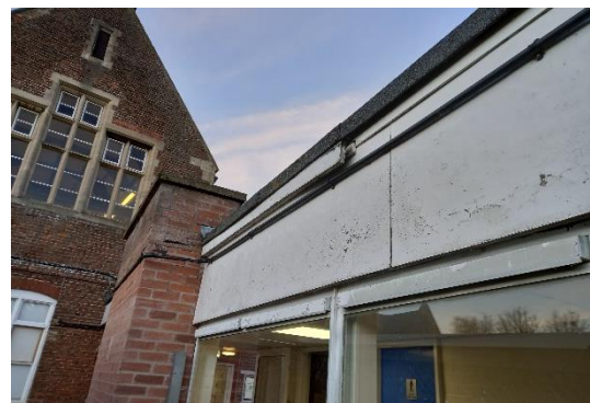
Figure: 12 Location: English Block Defect: Aged and life expired steel windows & timber fascia board
