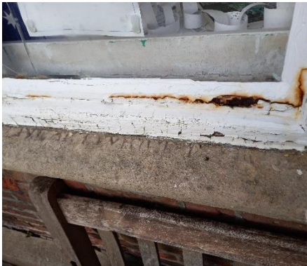
Figure: 7 Location: Original Building Defect: Further evidence of prolonged timber rot to timber windows
