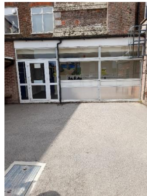
Figure: 10 Location: Original Building Defect: Aged and life expired steel windows
