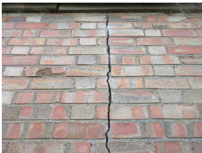
Photograph # 11 (Main 'Stable' Barn - Localised Cracking to Rear Elevation)
