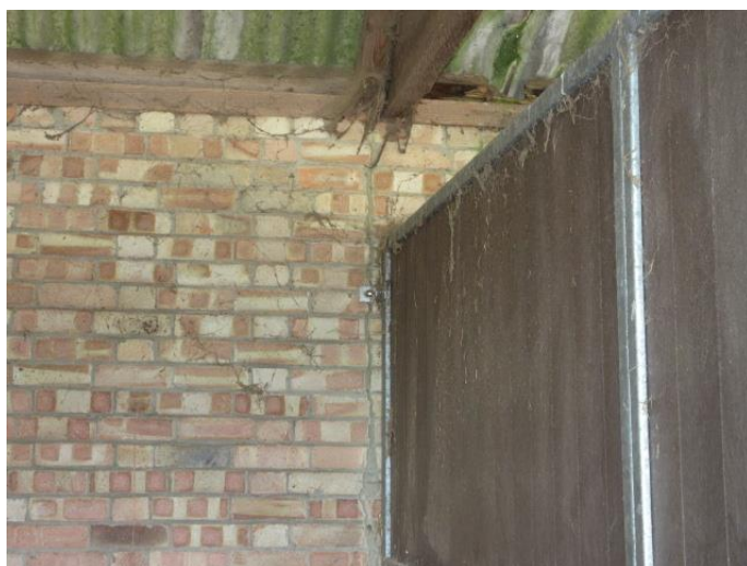
Photograph # 12 (Localised Cracking to Rear Elevation - Internal Brickwork – Crack Formerly Repaired)
