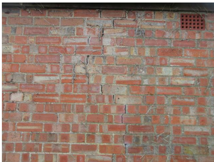
Photograph # 13 ('Store' Barn - Localised Cracking to Rear Elevation)
