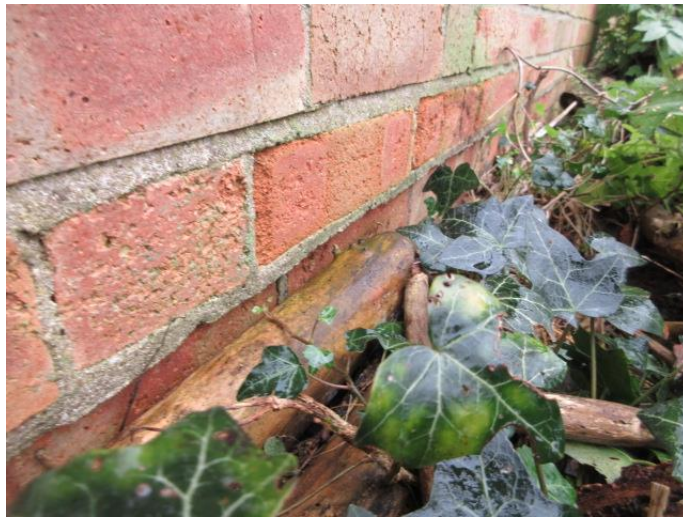
Photograph # 16 (Main 'Stable' Barn – Rear Masonry Panel – Horizontal movement on DPC)
