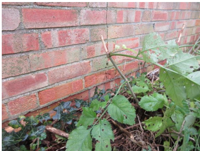
Photograph # 15 (Main 'Stable' Barn – Rear Masonry Panel – Horizontal Movement on DPC)
