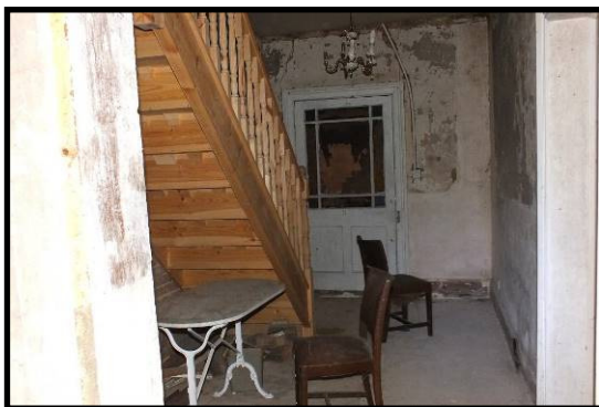
Later replacement staircase in the hallway that detracts from the character of the hall
