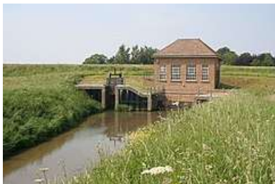
Lord's Drain pumping station was built in 1962 and pumps into the River Welland.
