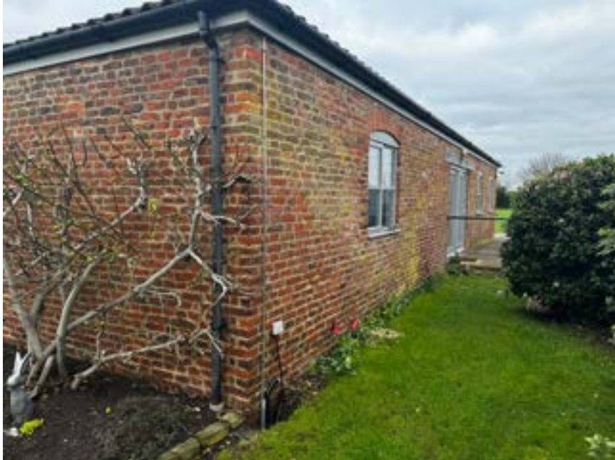
Image 2.0: View of Structure with Fig tree to elevation. Pit at corner return of building allowed for partial inspection of foundations.
