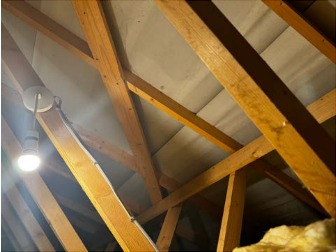
Image 5.0: Internal view of attic void, with breather membrane to gangnail trusses. Insulation clearly visible in image
