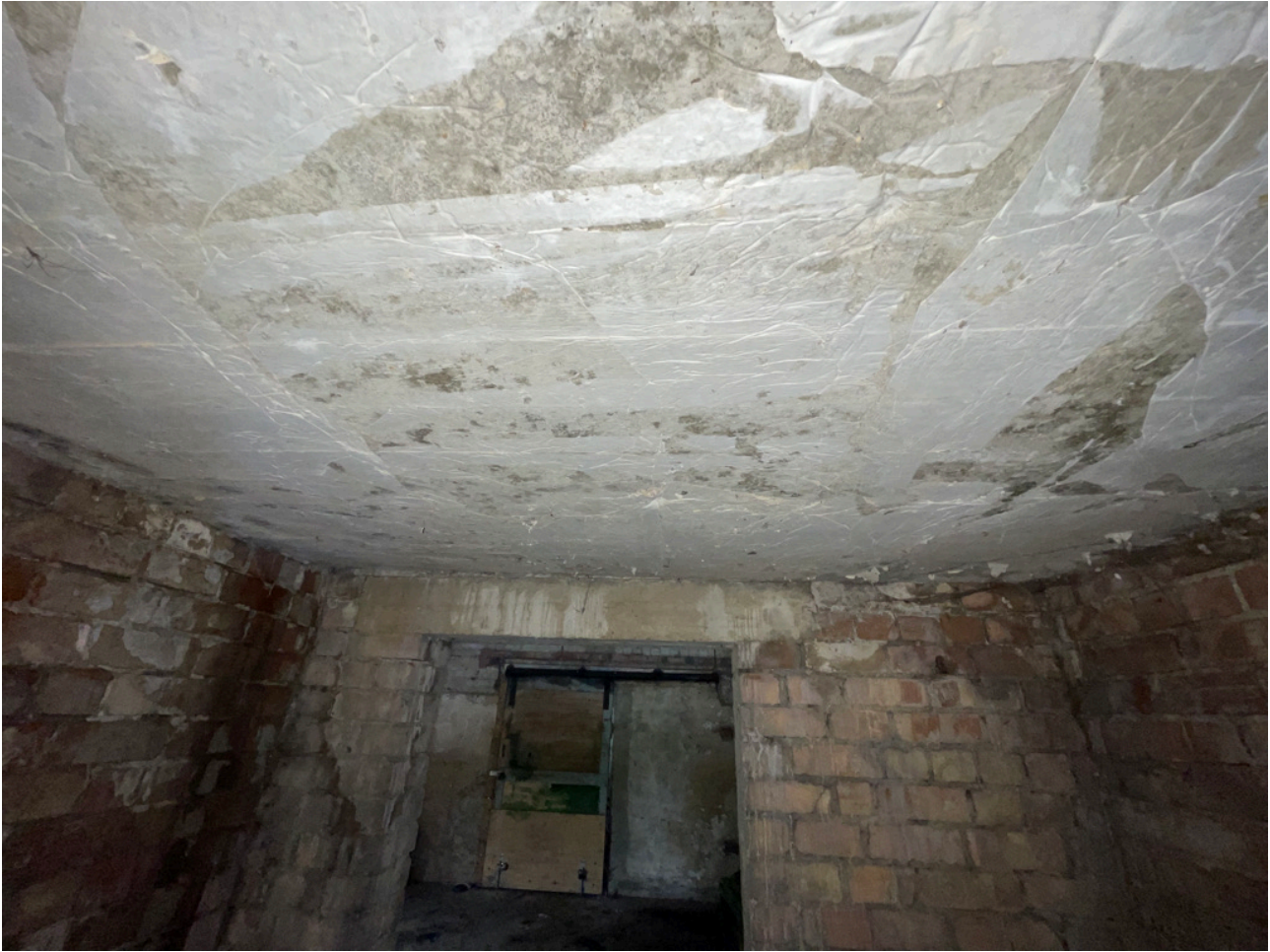
Image 18.0: water ingress to lintel set to head of doorway. Note polythene to underside of concrete slab, potentially reflective of a release mechanism for formwork to the cast-in-situ slab.
