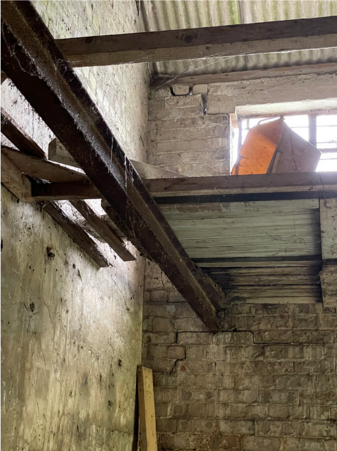
Image 15.0: Crack to masonry on side elevation, local to single storey structure.
