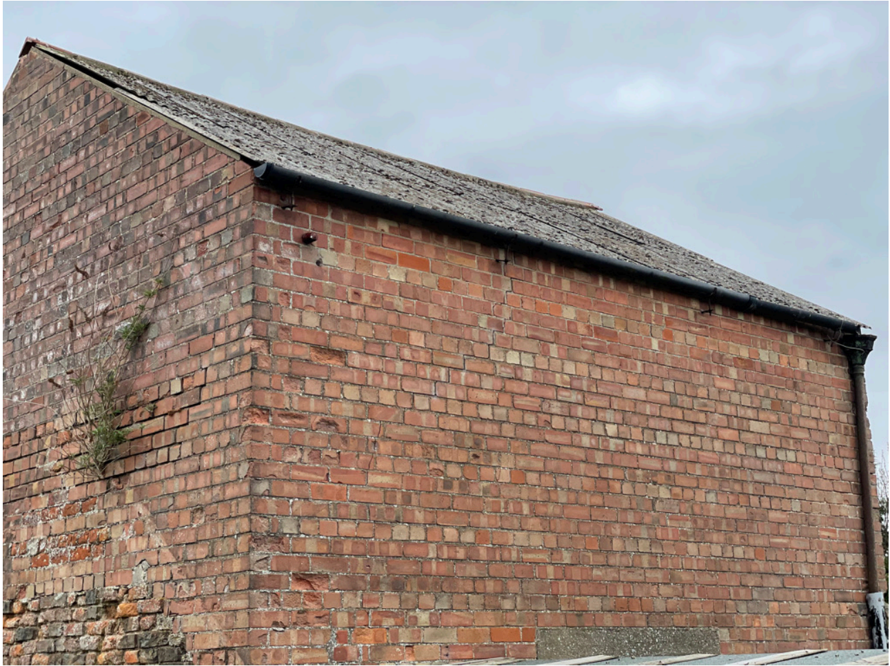
Image 14.0: Spalling to external brick faces
