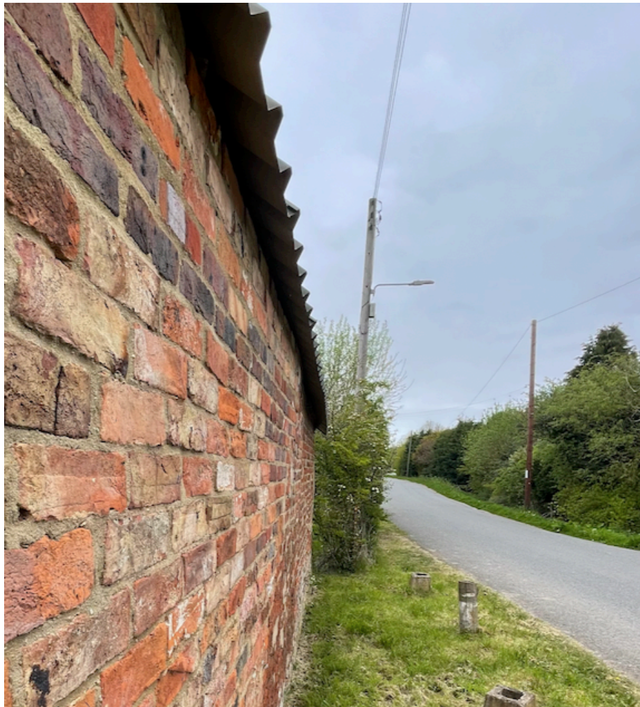
Image 11.0: Head of masonry deviating outward, local to weaker arch location
