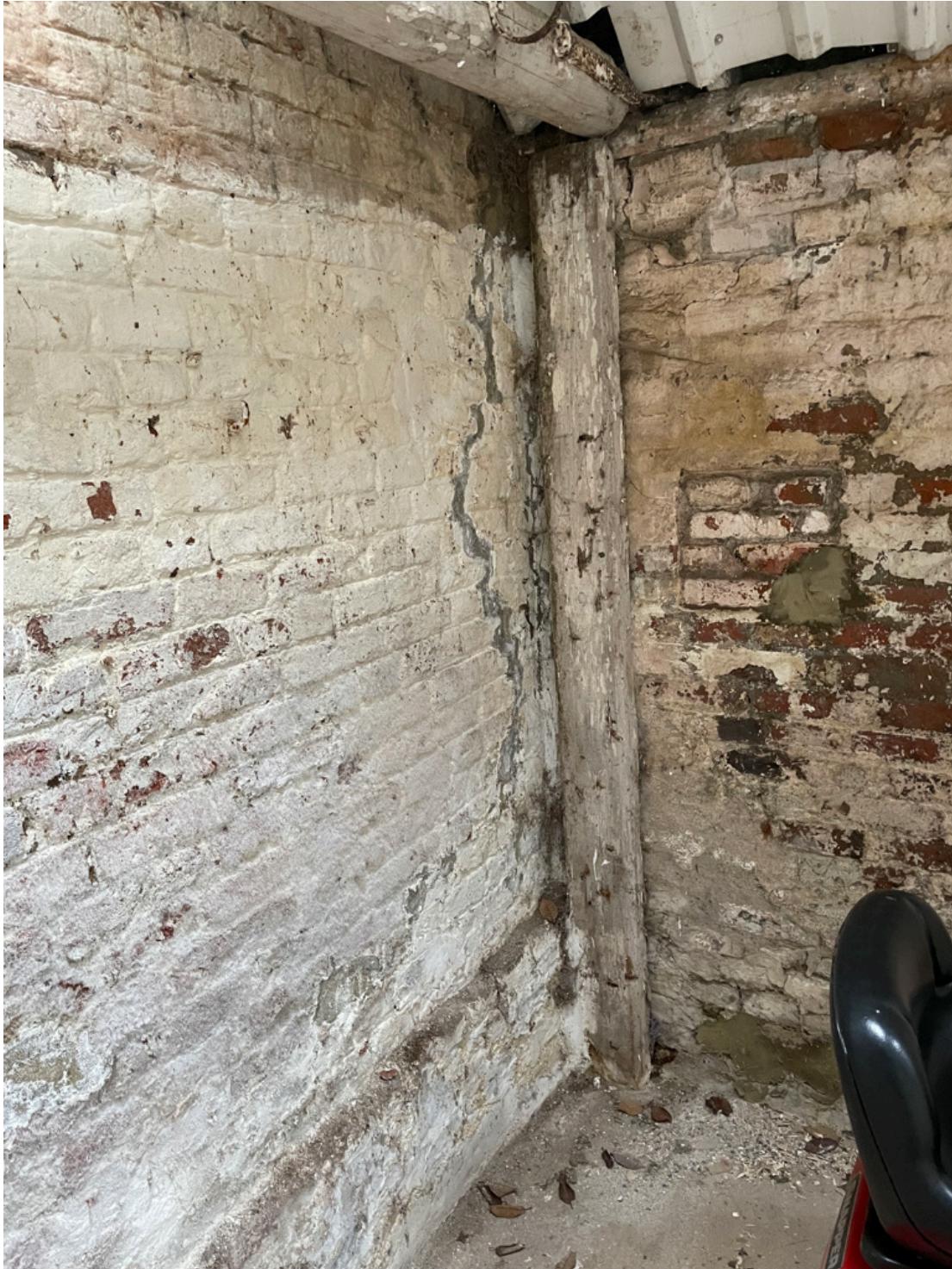
Image 8.0: Crack to rear gable
