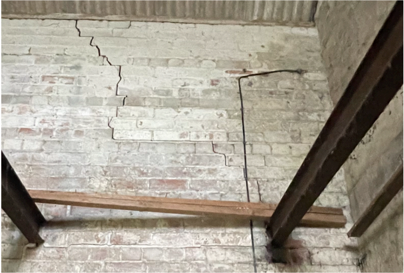
Image 16.0: Stepped cracking to opposite side elevation
