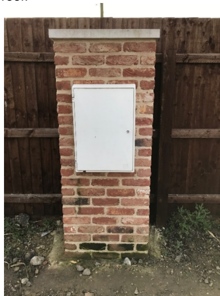
The Existing Electricity Meter.
