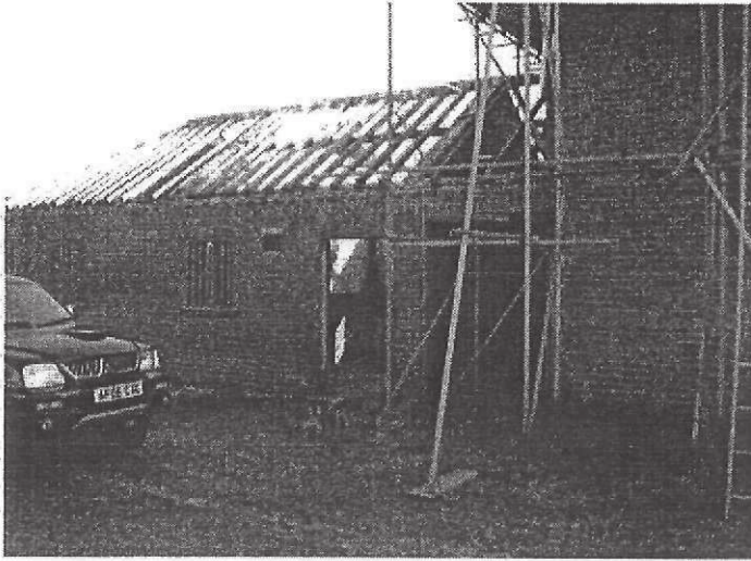
12. North wall of the main barn and North wing. Note the remaining rafters to the wing, which act as props to the remaining masonry.
