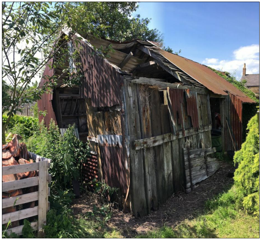
View - 01 Existing Collapsing Barn
