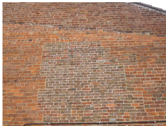
Fig. 06 – Dissimilar materials on the east gable.
