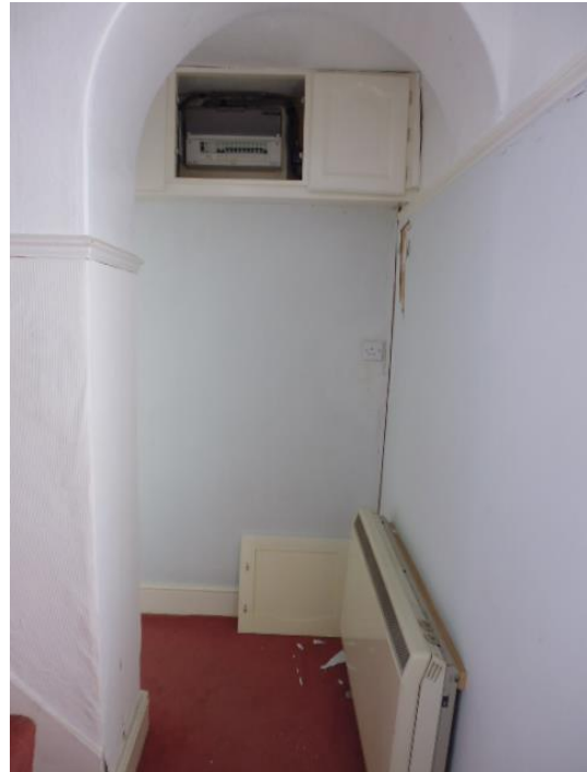
Fig. 14 – High level electric box cupboard.
