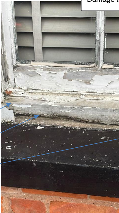
Damage to cill and transoms
