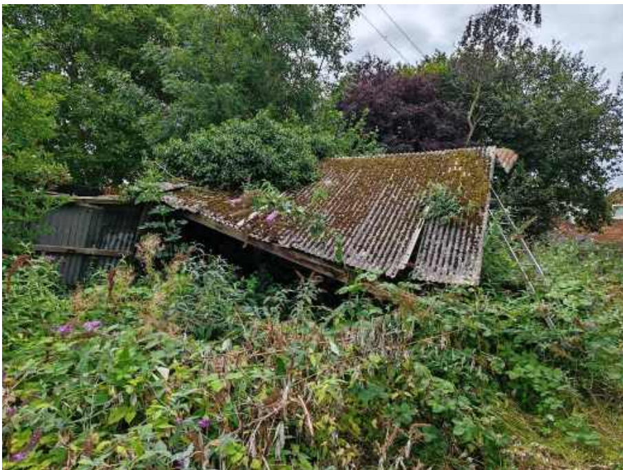
Site walkover photo: 3 Date: 05 Aug 2024 Photo direction: South Description: View of dilapidated farm building (cattle shelter) and overgrown vegetation
