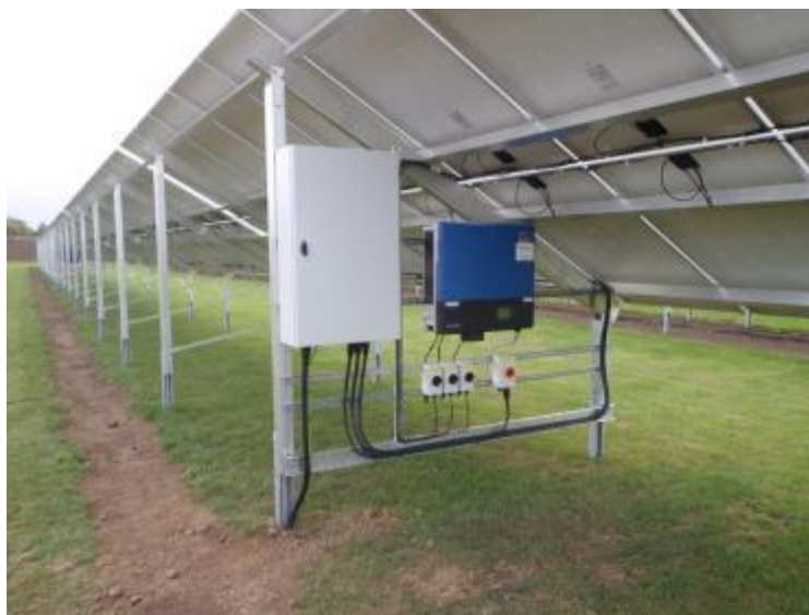
Fig. 3 Example of frame mounted enclosure and inverter
