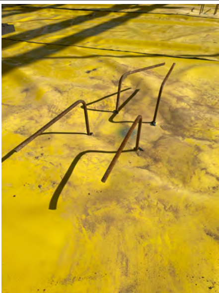
Steel fixings penetrating the membrane that have not been sealed.
