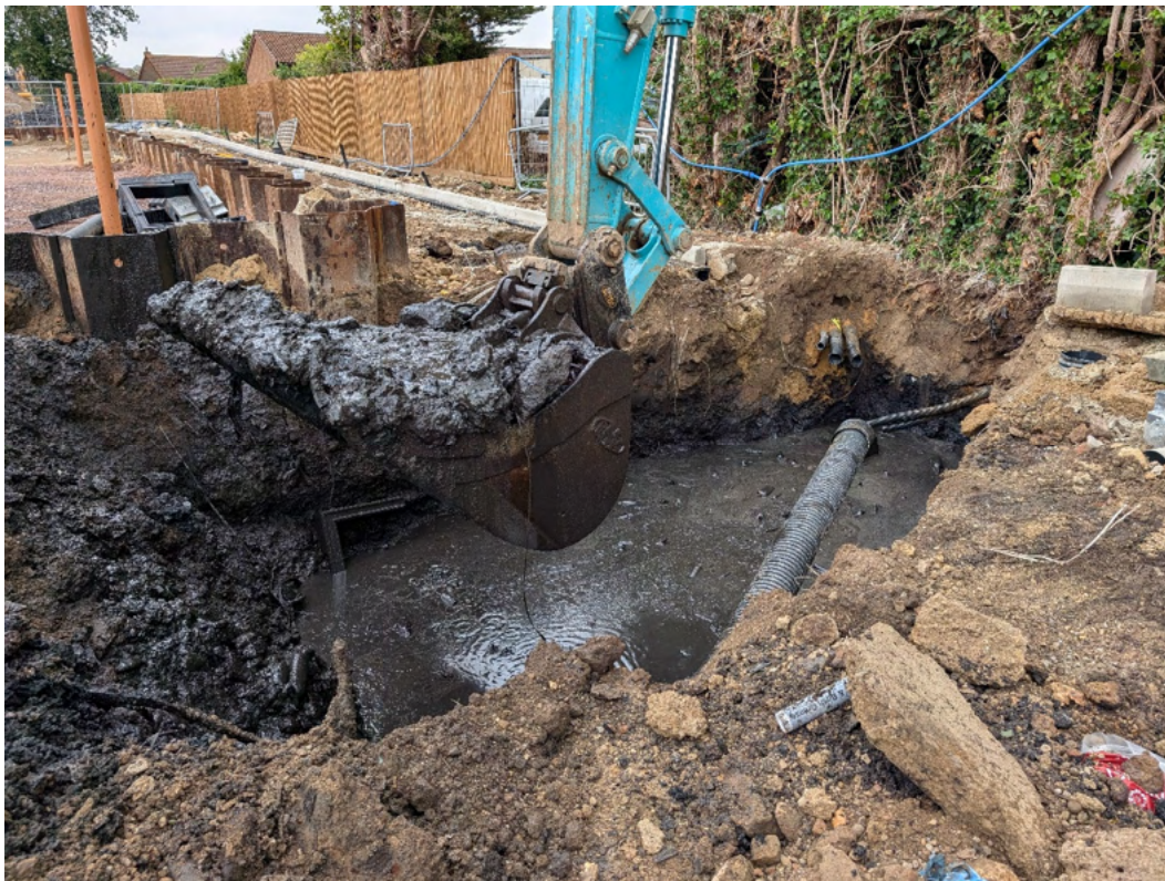
Delineation of former pond material (Water Ingress)
