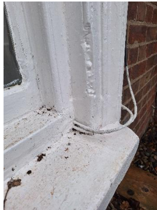
Existing timber windows in a deteriorating but repairable condition
