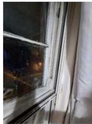
Existing timber windows in a deteriorating but repairable condition. Secondary glazing internally.
