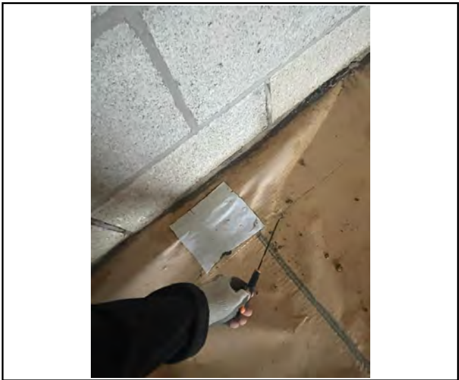
Pick and probe test carried out to hot
