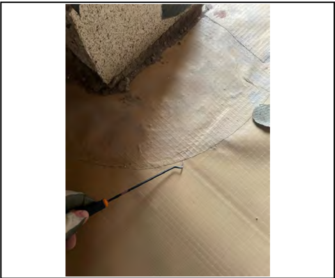
Additional pick and probe test carried
