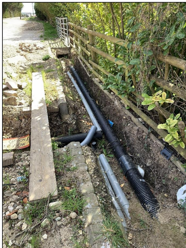
Photograph 4 – Exposed piped section of watercourse with lateral connections along the northern site boundary, looking east. Photograph taken by officers: 14/04/2026.
