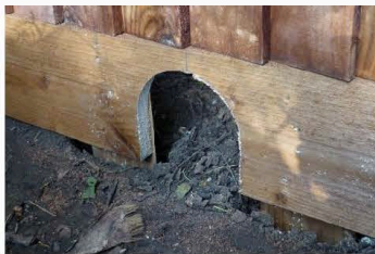
Hole in a timber fence panel
