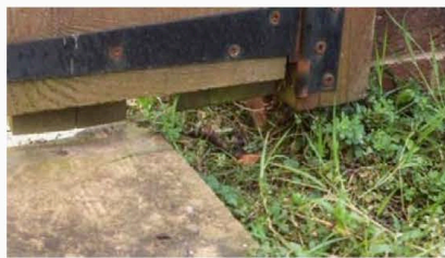
Gap under a gate
