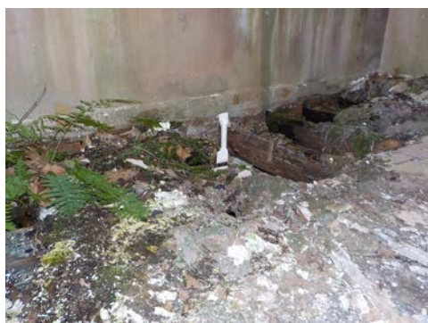
Photo 19 – Collapsed timber first floor
