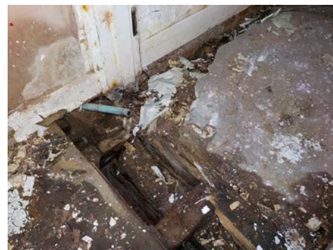
Photo 15 – Collapsed floor in rear extension
