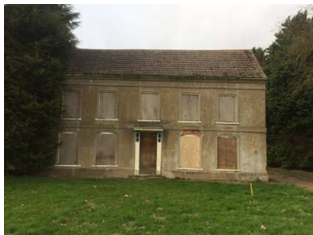
Photo 1 – Front elevation with Leylandii Cypress close to west gable
