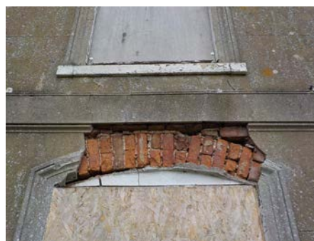
Photo 4 – Render missing over front window and masonry bearing onto timber windows
