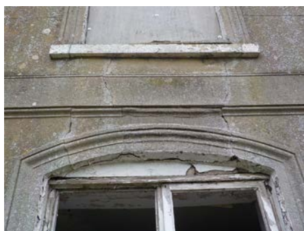
Photo 3 – Render cracking between windows. Masonry bearing onto timber window
