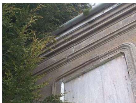
Photo 5 – Diagonal cracking above first floor window
