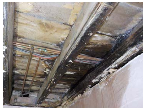
Photo 18 – Rotten timber first floor to rear extension
