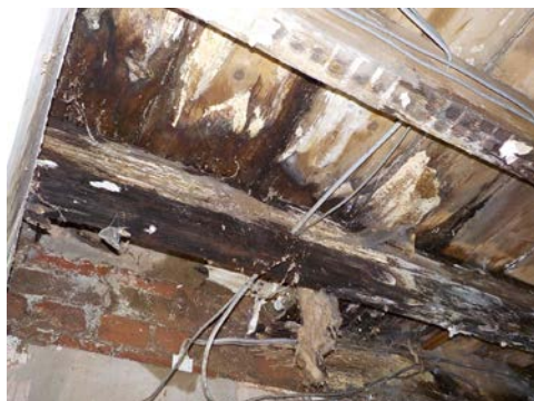
Photo 17 – Rotten timber first floor
