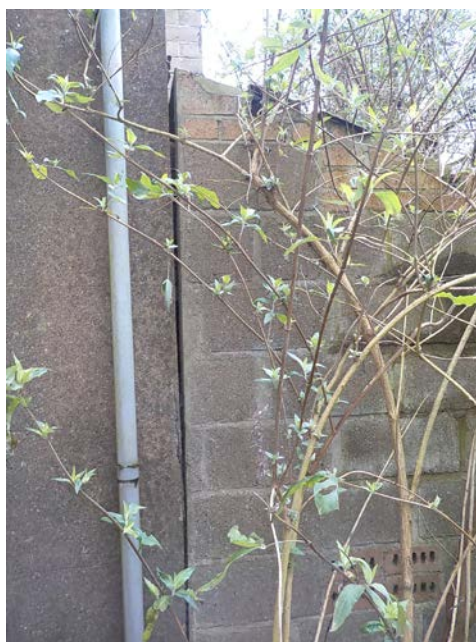
Photo 12 – Rotational movement visible between sections of masonry
