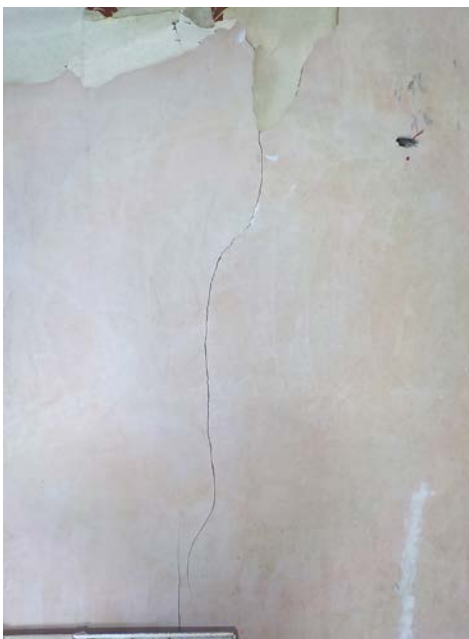
Photo 13 – Vertical cracking in the reception room
