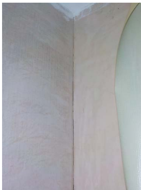
Photo 16 – Vertical cracking visible in lounge south west corner
