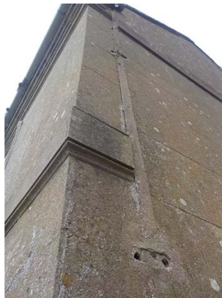
Photo 9 – Vertical cracking at corner junction between front panel and gable wall
