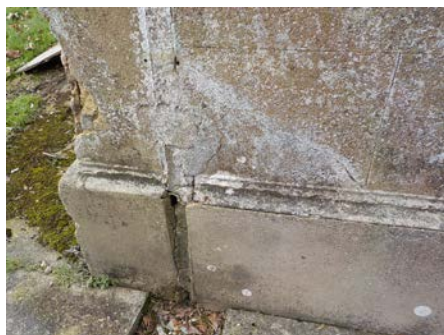
Photo 8 – Diagonal corner cracking, historically repointed
