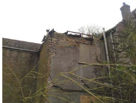
Photo 11 – Collapsed masonry section
