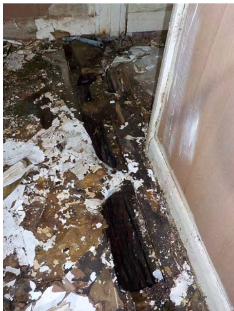
Photo 14 – Rotten collapsed timber floor in hall
