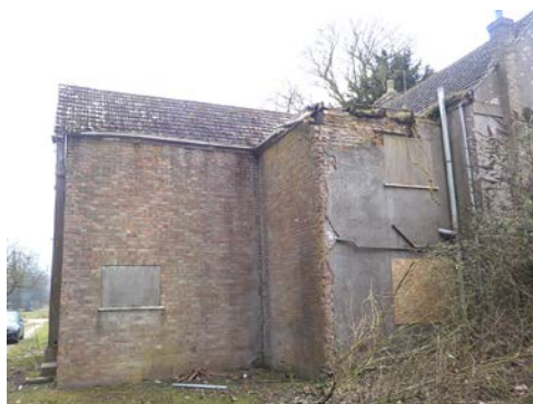
Photo 10 – Part rear elevation, collapsed timber roof and masonry panel
