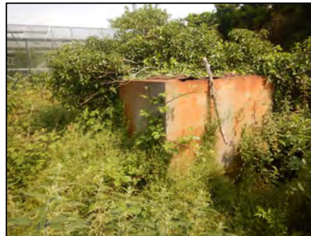
Photo 15 Corroded empty bulk storage tank
