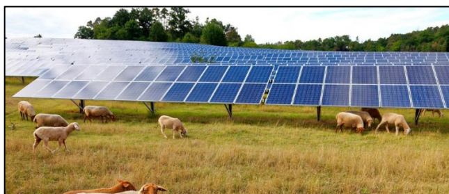
Figure 3.3: Typical Static South facing Solar Arrays
