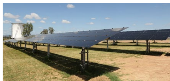
Figure 3.4: Typical Single Axis Tracking Solar Arrays
