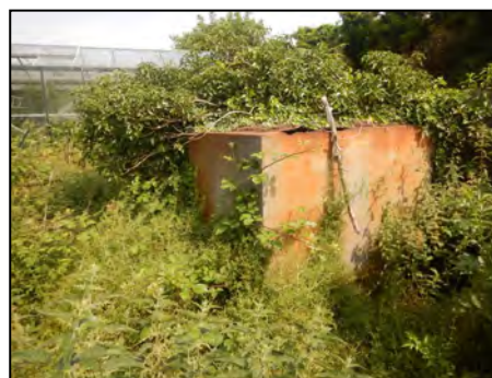
Photo 15 Corroded empty bulk storage tank
