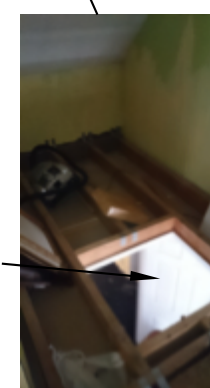
existing staircase position boarded over by previous owners
