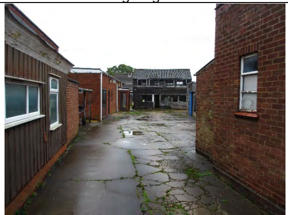
Photo 4: View of sales room on left and workshop/ store at rear of picture
