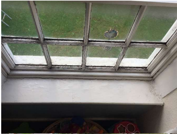
5. Window in right hand bedroom - to be repaired, remove rotten timber and replace in matching softwood.
