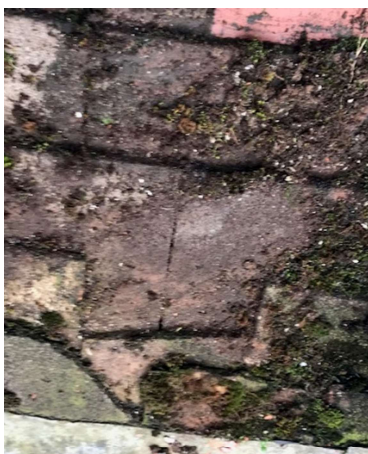
9. Damaged roof tiles
