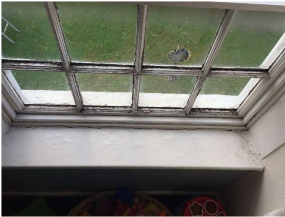
13. Window in right hand bedroom - to be repaired, remove rotten timber and replace in matching softwood.
