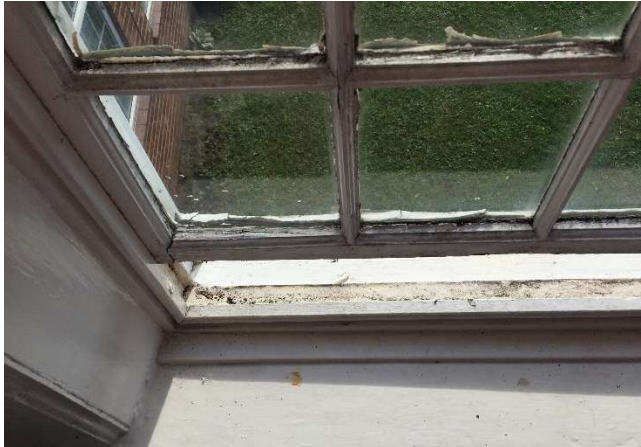
11. Window in right hand bedroom - to be repaired, remove rotten timber and replace in matching softwood.
