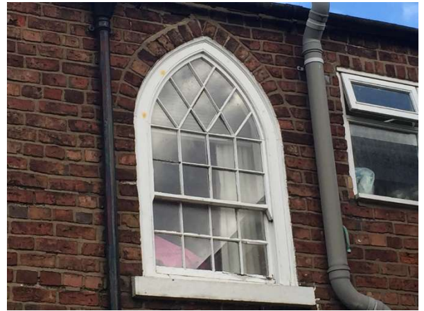
8. Window in right hand bedroom - to be repaired, remove rotten timber and replace in matching softwood.
