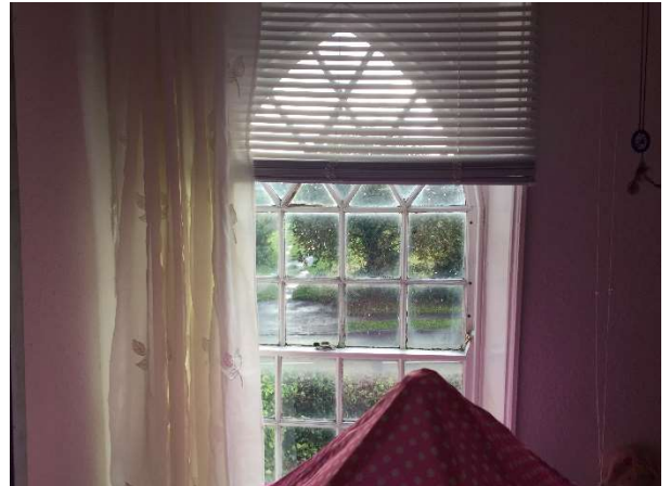
6. Window in right hand bedroom - to be repaired, remove rotten timber and replace in matching softwood.
