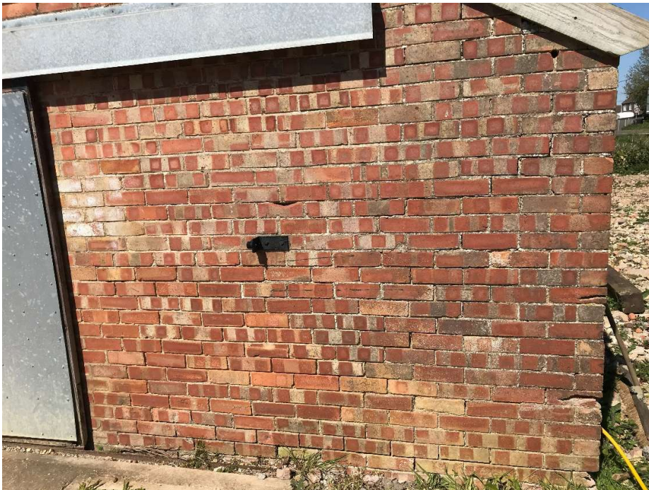
Photo 10. East-side of Southern Gable End Elevation. Typical weathered masonry and hairline cracks
