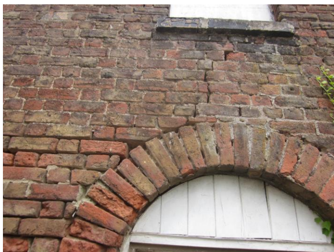
Photograph # 11 (Typical Distorted Arch / Masonry over Arch)
