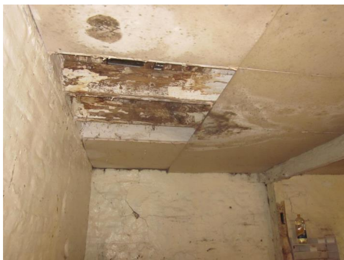
Photograph # 21 (Underside of First Floor – Water penetration / decay)
