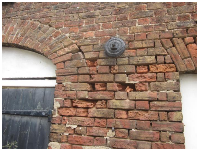
Photograph # 10 (Typical Perished Masonry Arch / Pattress Plate)
