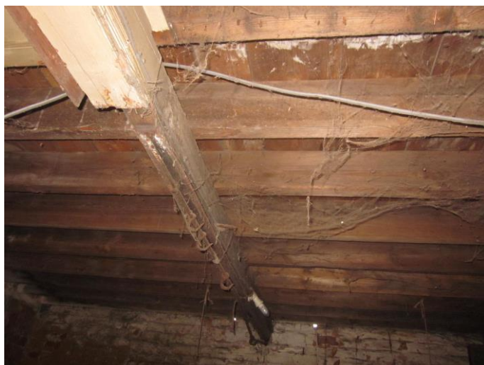
Photograph # 19 (Underside of First Floor – Undersized Beams)
