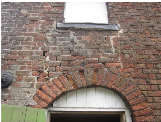
Photograph # 9 (Typical Distorted Arch / Masonry over Arch)
