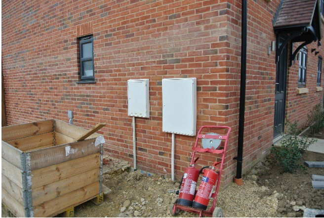
Typical meter box installations. 06.04.2022
