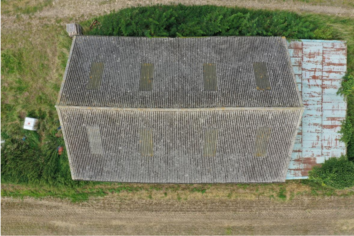
Ph. 5 Aerial view of the barn showing suspected ACM to the roof.
