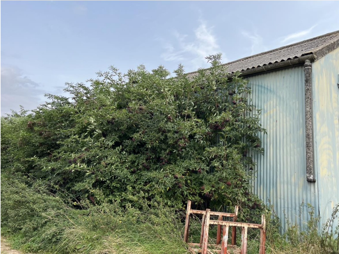
Ph. 6 Side view of the barn showing suspected ACM to the rainwater goods.
