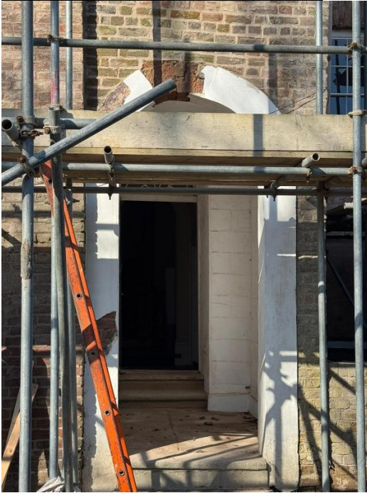
Photographs of Brickwork below Render
