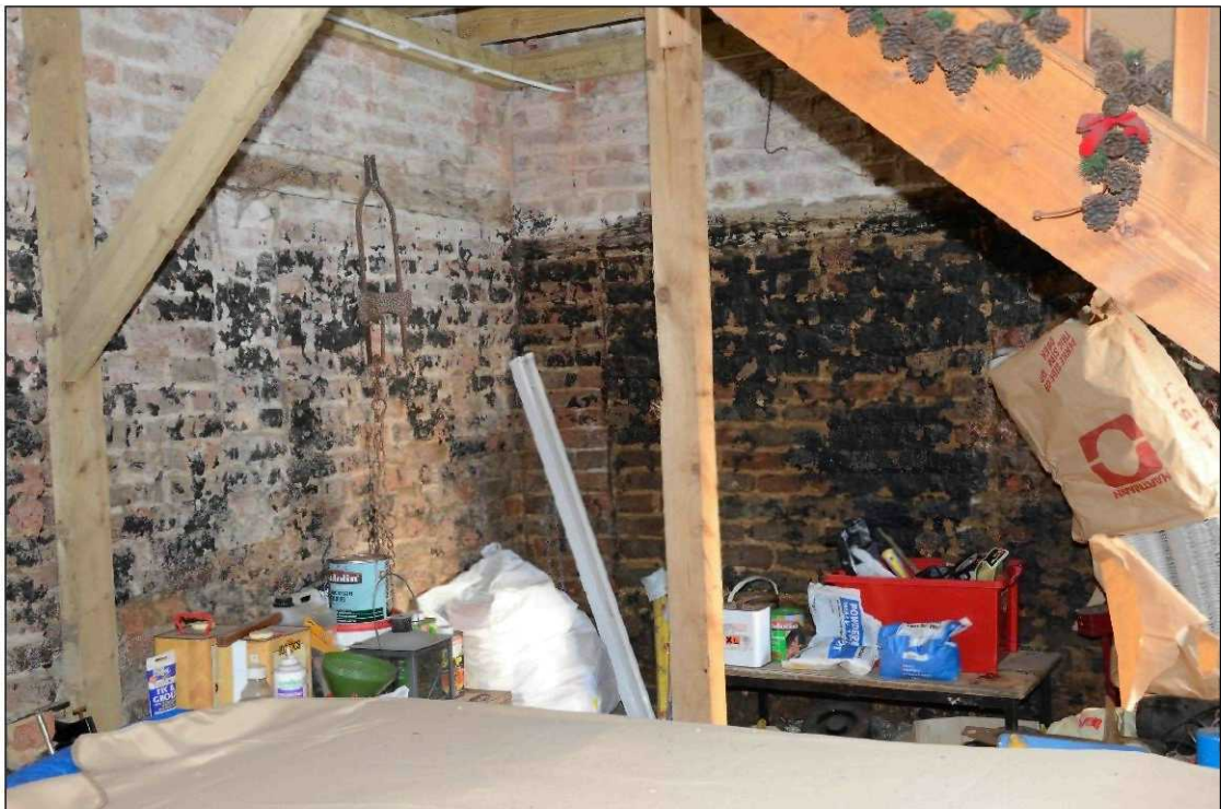
Plate 20: Building 1: blocked ventilation slot (left) and doorway (right), looking southwest
