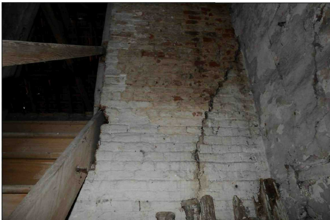
Plate 42: Building 2, crack in 'granary' wall as seen from covered entrance, looking south
