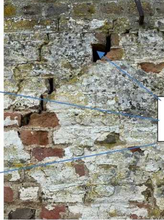
Timber Lintel Failure Causing cracking
