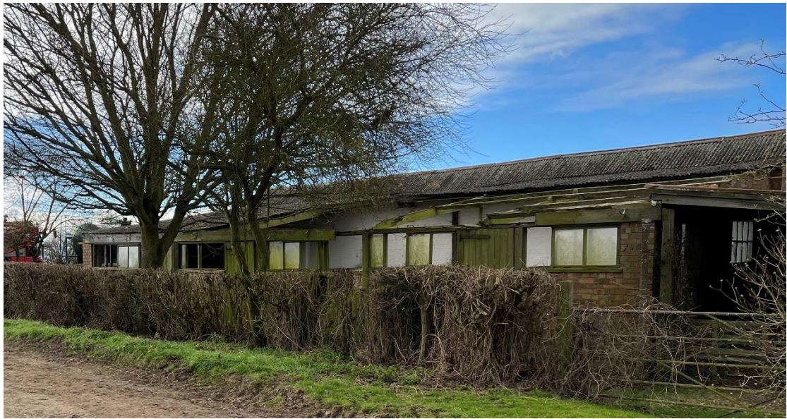
Dilapidated lean-to on eastern side.
